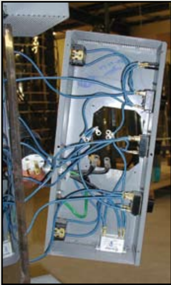
Electrical box without kiln sitter
